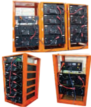
Energy Storage System (ESS)
